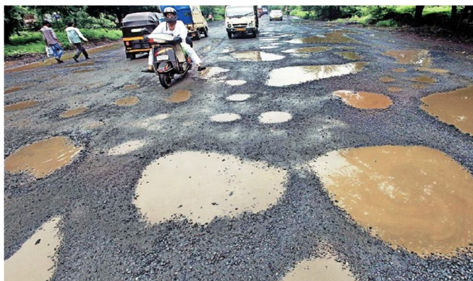
Figure1. Potholes present on the roads
